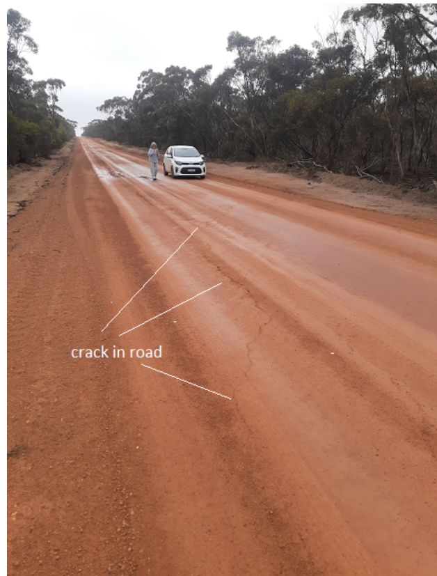
Figure 8. Crack in north-south road east of Gnowangerup
