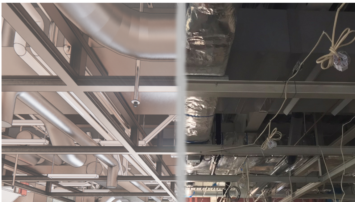
Figure 31: Seismic Restraint 3D Model compared with the physical installation on site. (Beca).
