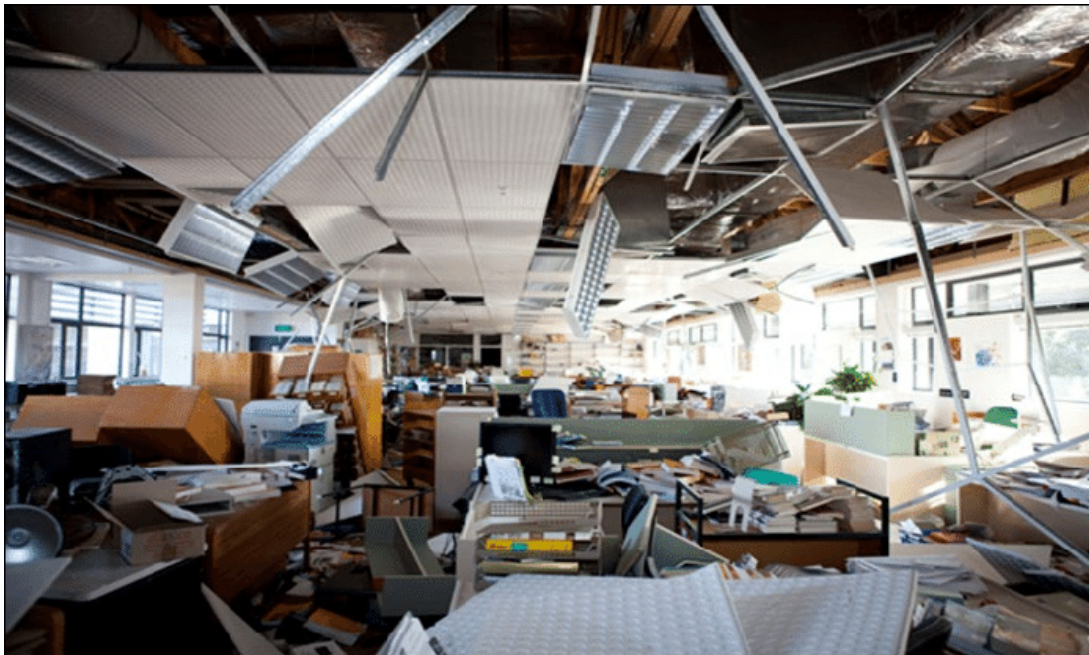
Figure 1: Damage to non-structural elements observed in the Canterbury earthquakes. (Dhakal, 2010).
