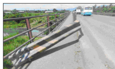
Damaged Kerb on Guard Fence
