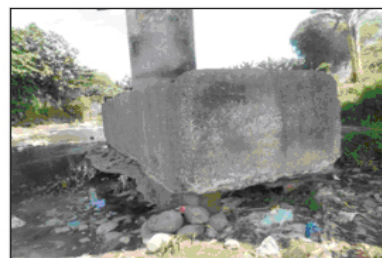
Scoring around Mid-Span Pier Foundation
