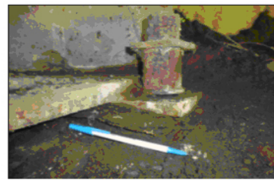
Corrosion of Bolt Connection at North Abutment
