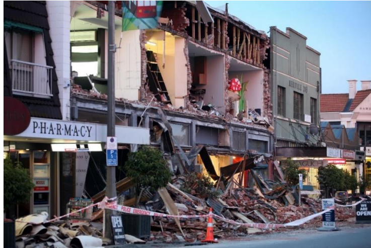
Figure 7 Collapsed URM facades in Christchurch. Photo: Alamy.
