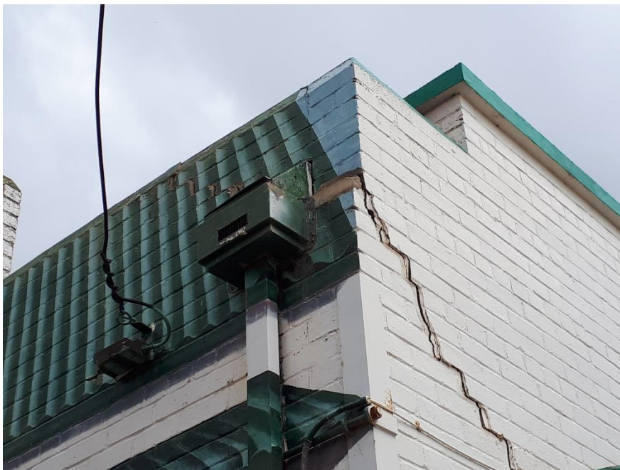
Figure 7 Damage from 2021 event over repaired damage from previous event. Previous angle iron strengthening on corner.
