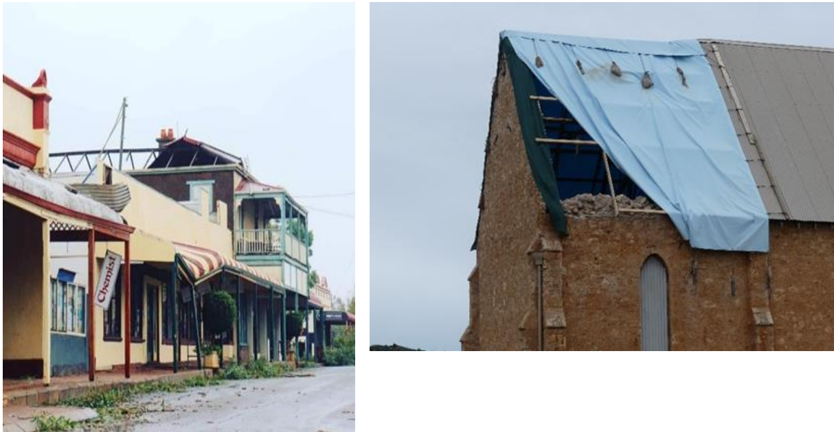
Figure 1 Wind damage caused by Severe Tropical Cyclone Seroja which passed over south-west WA in April 2021 (courtesy DPLH)
