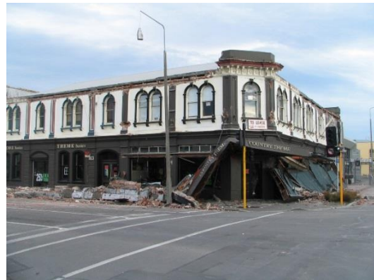
(b) Parapet with no ties back to roof
