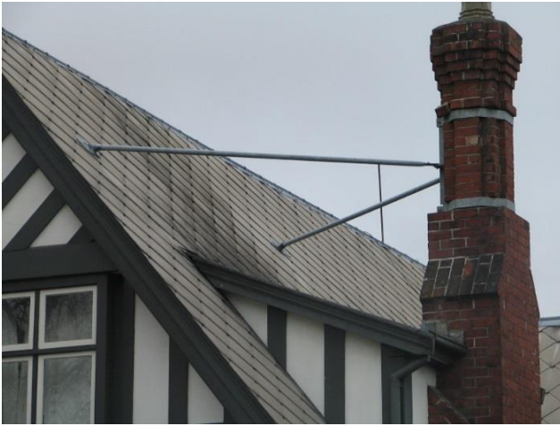
Figure 2: Successful chimney retrofit survived the M_w7.1 September 2010 earthquake.
