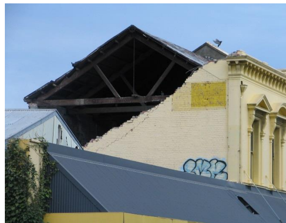
(b) Unsecured gable wall failure
