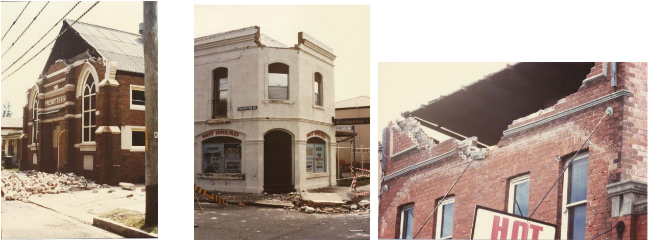
Figure 1. Damage from face loading (Page)
