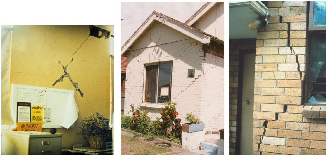
Figure 2. Damage from in-plane loading (Page)
