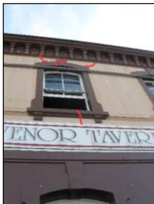
(e) Cracking in exterior façade, after 4 September 2010
