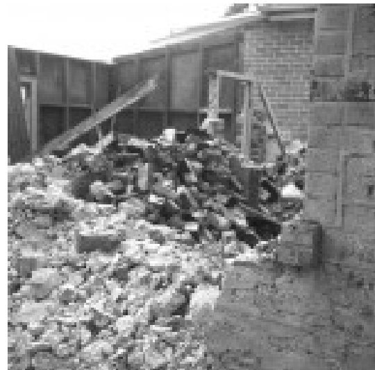
Figure 1: Failure of masonry to housing, Adelaide. Photograph courtesy AEES.
