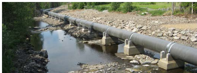
Fig. 4. A typical above ground pipeline
