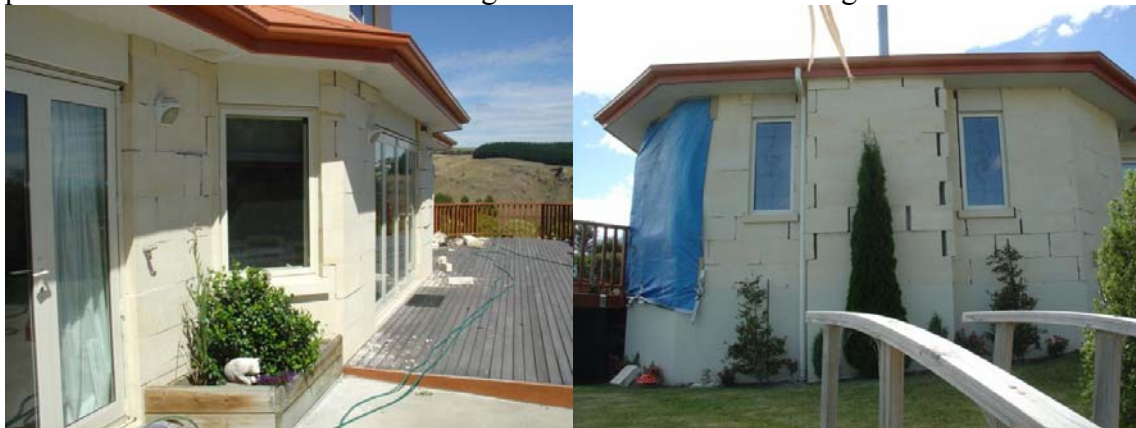
Figure 7 Two storey light steel frame house with Oamaru stone cladding [T Just]
