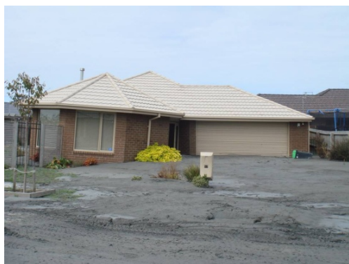
(c) Ground instability [M Pender]
