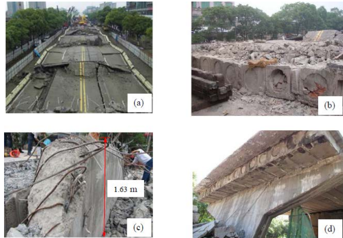
Fig. 4. Hongqi Viaduct after collapse: (a) overview, (b) collapsed slabs, (c) remaining pier (#109) and (d) pier #101.
