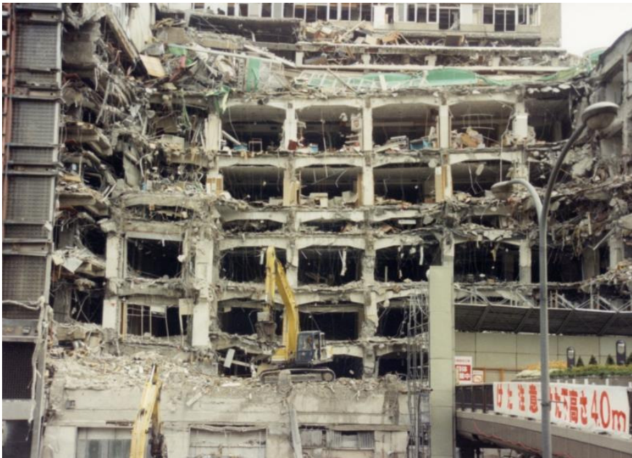
The Kobe earthquake (Photograph courtesy John Woodside)
