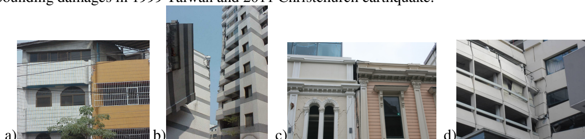
Fig. 1. Observed pounding damages between adjacent structures in Taiwan (a&b) and Christchurch (c&d)
