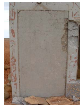
Figure 7. Observed spalling at front face of tested panel
