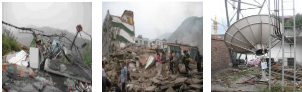
(a, b) Damaged unreinforced masonry and equipments (c) Satellite dish under the tower [C, 7]
