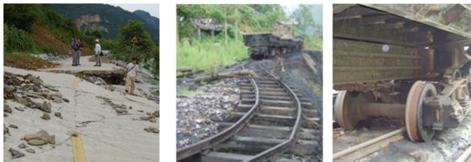
d) Failure of highway foundation (e) damaged railing track (f) carriage off the track
