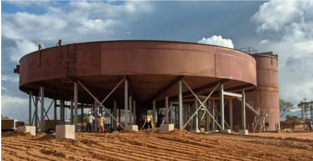
Figure 1: Typical thickener tank installation
