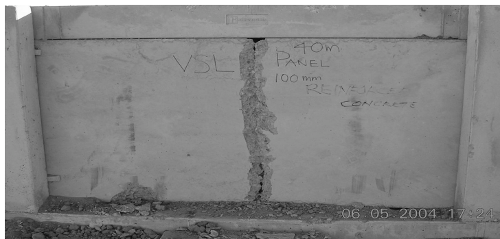
Fig 3. NSC panel after explosion (after Ngo 2005)
