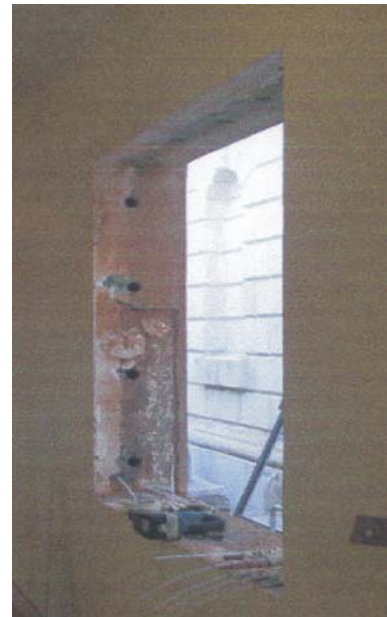
Figure 1: Typical retrofit project in brick masonry drilled and ready for blast proof window installation
