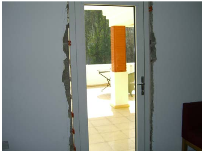
Figure 4: Rotary percussion drilled holes located too close to the masonry surface causing extensive spalling around perimeter of blast proof door.
