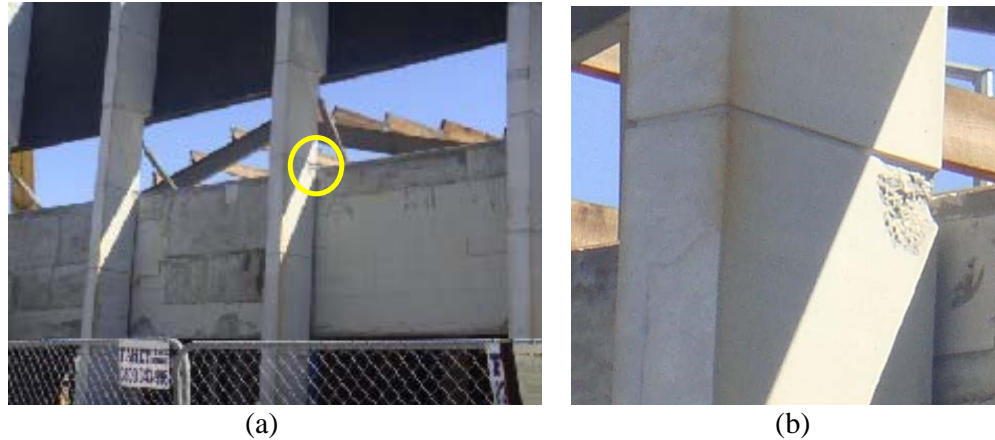
Figure 2: Damage due to relative movement between columns and floor in the CBD. (a) Overview and (b) pounding location.
