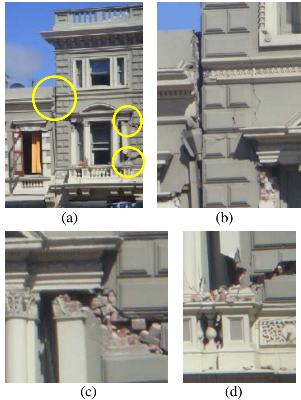
Figure 5: Pounding induced damage to adjacent buildings in the CBD. (a) Adjacent buildings, (b) damage at the pounding location, (c) induced damage at the top and (d) at the right corner of the right window.
