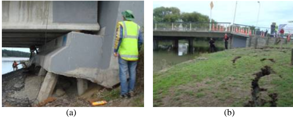
Figure 6: Typical damage to road bridges outside the CBD during the 2010 Darfield Earthquake: (a) Bridge Street bridge; and (b) Avondale Road bridge
