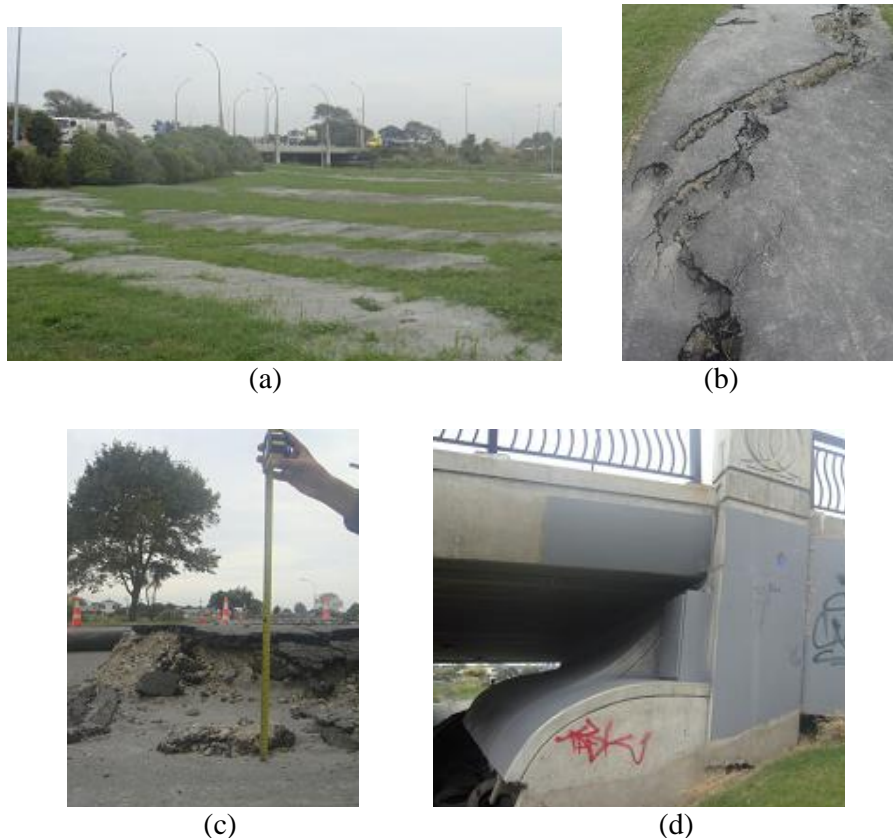
Figure 7: Damage to the ANZAC bridge and surroundings due to the 2011 Christchurch Earthquake: (a) sand boils on local site; (b) damage to walkway beneath the bridge; (c) relative ground movement around a manhole next to the bridge; and (d) damage to bridge abutment.
