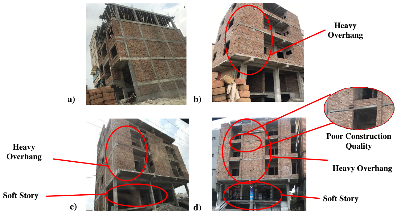
Figure 2: RCC Structures: a) at no risk, b) at low risk, c) at moderate risk, and d) at high risk
