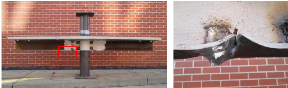
Figure 9. Steel fracture observed in specimen CS-5.
