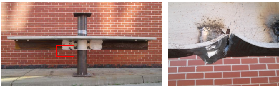
Figure 9. Steel fracture observed in specimen CS-5.
