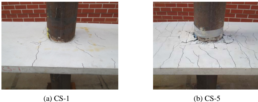
Figure 14. Concrete cracks and crushed concrete in slabs.
