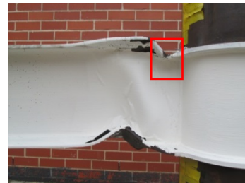
Figure 6. Buckling of the beam and fracture of the weld seam.
