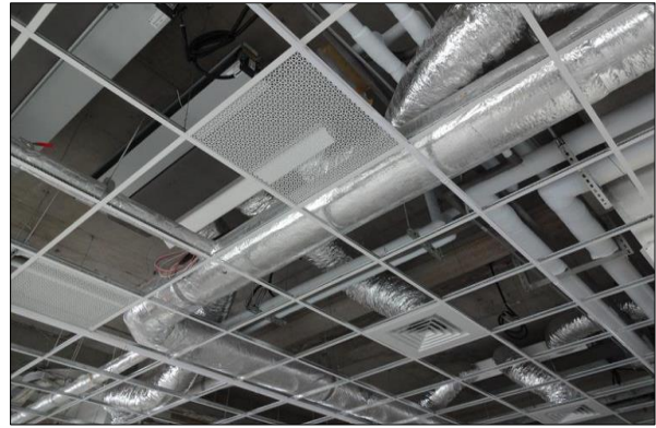
Figure 2. Unfavorable installation condition
