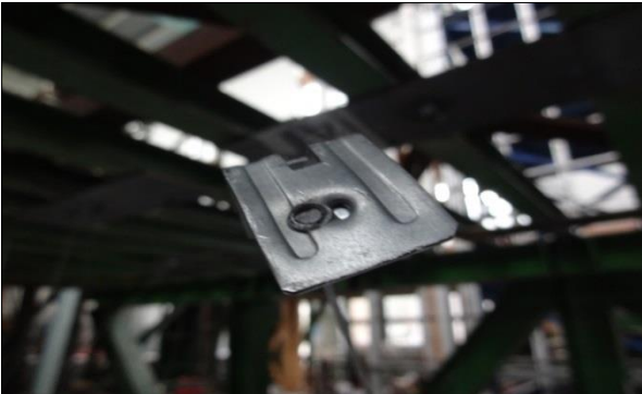
Figure 15. Failure of hanger wire
