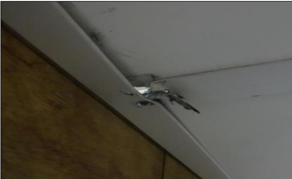
Figure 13. Failure of perimeter connection
