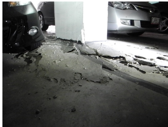
Figure 1: Punching shear failure in Grand Chancellor building, Christchurch
