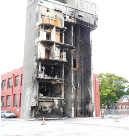
Figure 4: Failure of connection between diaphragm and core, CTV building, Christchurch
