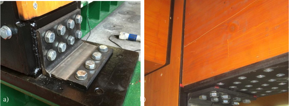
Figure 8: a) Fracture of dissipative angles at base and b) tension cracking of beam at first floor
