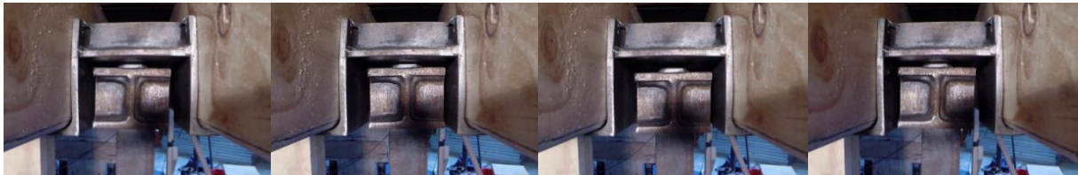
Figure 5 - Gap between corbel and inside of saddle bracket to accommodate bidirectional movement
