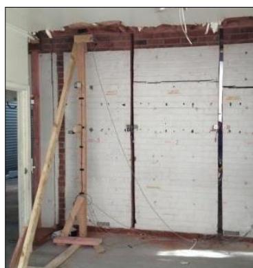
(a) Instrumentation framing at Auc-W3 after Auc-W1 and Auc-W2 have been tested and cracked
