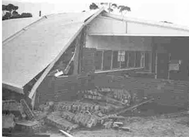
Figure 6: Damage in Cadoux Western Australia due to the M6.2 June 2, 1979 earthquake
