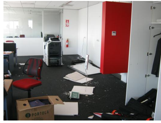
(d) Typical interior of office following 22 Feb 2011 earthquake [C Clifton]
