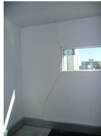
(b) Cracking to internal linings of window-box [C Clifton]
