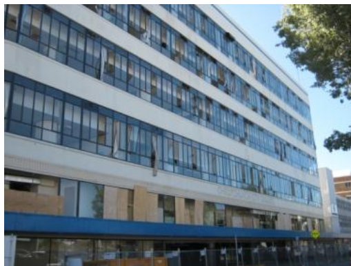
(a) Structural and claddings damage [J Ingham]
