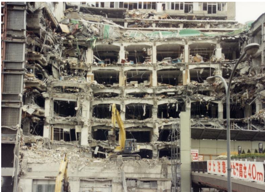
The Kobe earthquake (Photograph courtesy John Woodside)
