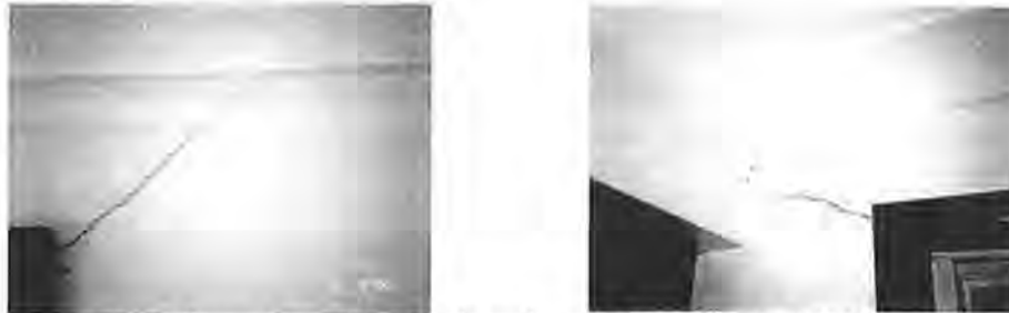
Figure 1: Typical diagonal cracking in plasterboard (Moore et al., 2002)
