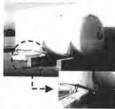
Figure 1. Rooftop tank failure, 1994 Northridge earthquake
