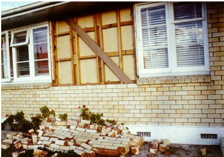
Figure 1 Example of brick veneer failure in the 1987 Edgecumbe earthquake
