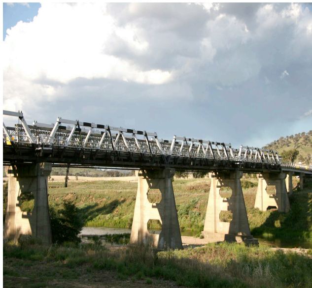
Tharwa Bridge, an iconic entrance to Namadgi National Park (photo Sabine Friedrich)
