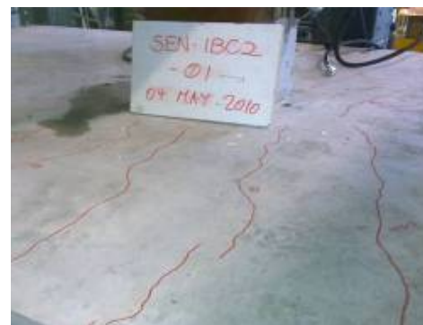
Figure 13 Crack of slab in specimen 3
