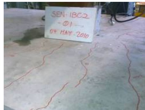
Figure 13 Crack of slab in specimen 3
