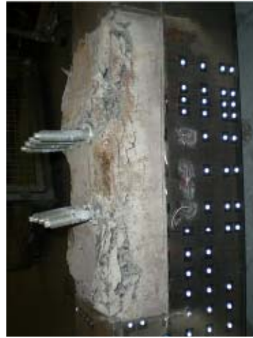
Figure 9 Concrete in square column
