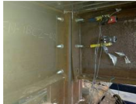
Figure 17 Flush endplate in specimen 4
