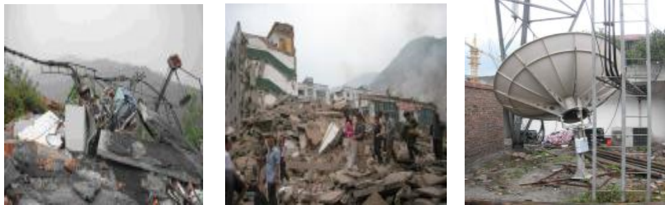
(a, b) Damaged unreinforced masonry and equipments (c) Satellite dish under the tower [C, 7]
