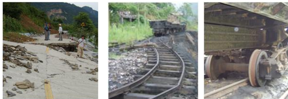
d) Failure of highway foundation (e) damaged railing track (f) carriage off the track
