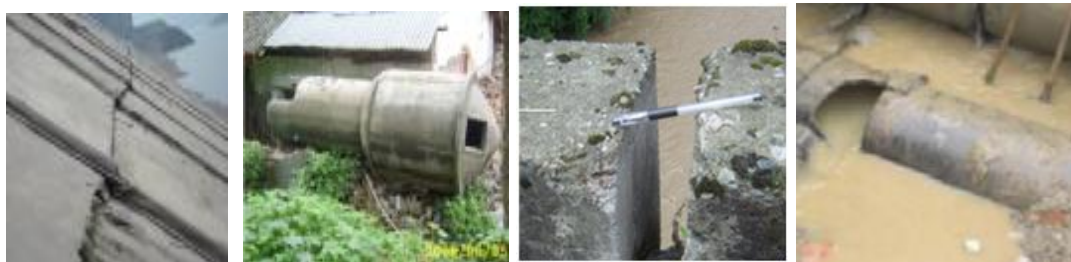
Fig.5. damaged water supply system
