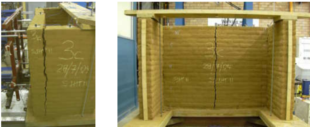
Figure 6a&b. Vertical corner cracking and mid-span vertical cracking of Specimen 3C (with horizontal mesh reinforcement) after shake table testing (Dowling, et al., 2004)
