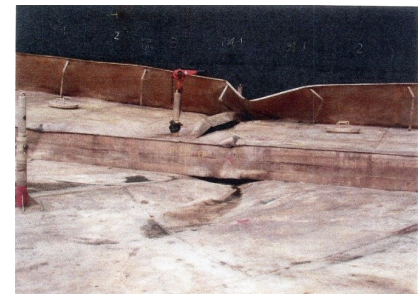
Buckling of pontoon
