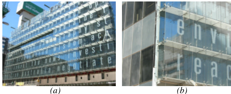
Figure 3 - Building One, butt jointed glass façade supported on “spider” corner fixings (a) general view of façade facing street, (b) close up of double skin glass.
