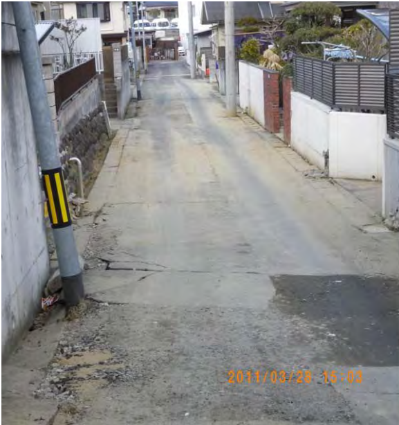
Fig. 10 Remains of liquefied sand at road surface in residential area where former water stream was filled with cut soil
