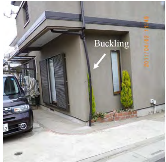
Fig. 29 Liquefaction-induced tilting (Kazo City)
