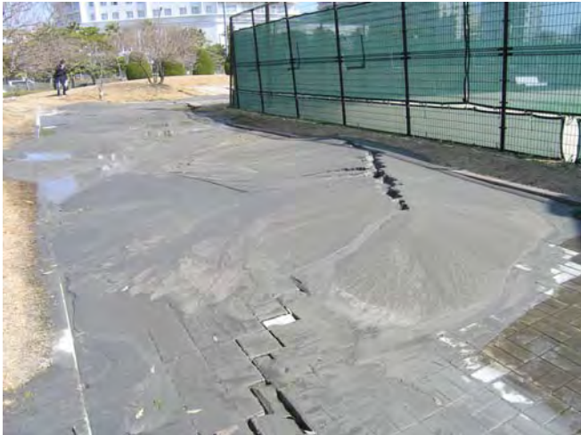
Fig. 16 Liquefaction and sand ejecta in Urayasu City
