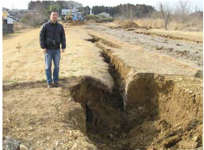
Fig. 12 Liquefaction-induced lateral spread and subsidence of Naka River levee
