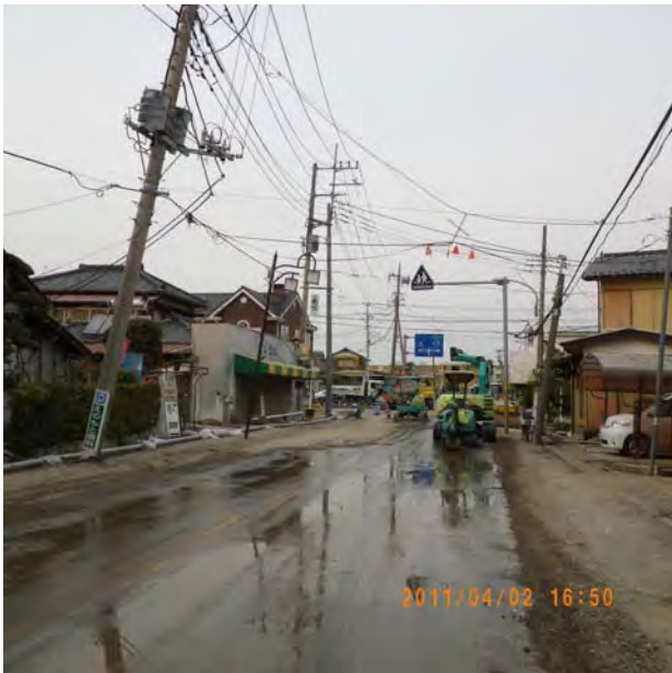
Fig. 27 Liquefaction in filled pond (Abiko City)
