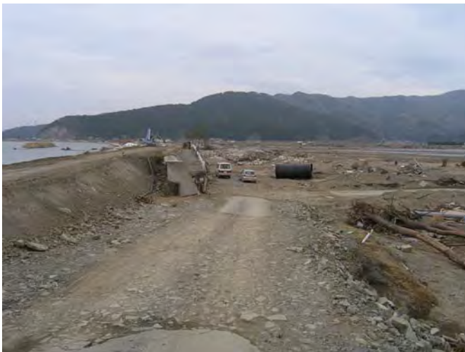
Fig. 7 Damage of Kitakami River levee that was directly hit by tsunami
