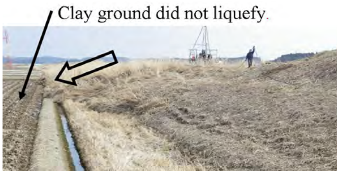
Fig. 14 Damaged levee resting on unliquefiable clayey subsoil (levee of Naruse River, north of Sendai)
