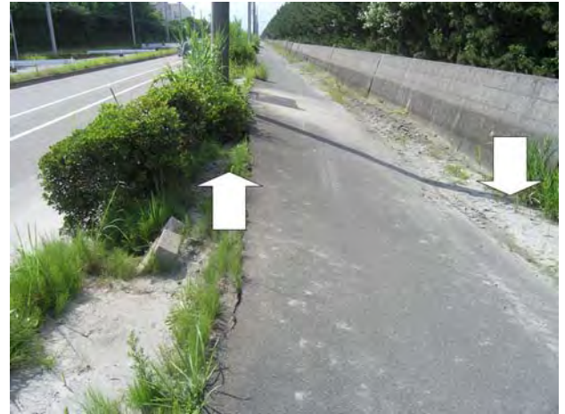
Fig. 23 Liquefaction-induced distortion of sidewalk
