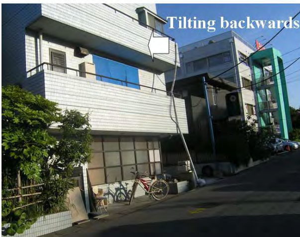
Fig. 21 Subsidence and floating of residential building
