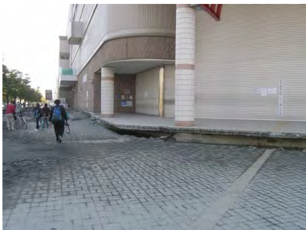
Fig. 18 Differential settlement between surface of liquefied ground and pile-supported building
