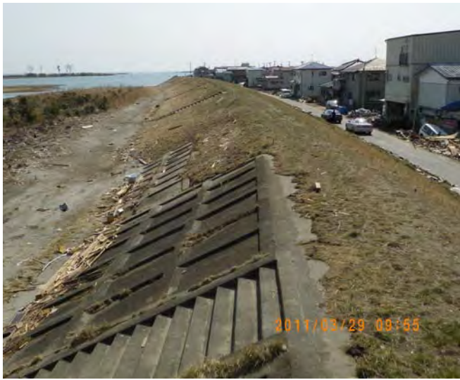
Fig. 6 River levee that survived tsunami in spite of overtopping (Natori River at Yuriage)
