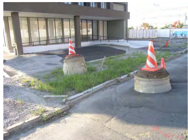
Fig. 20 Floating of a series of manholes
