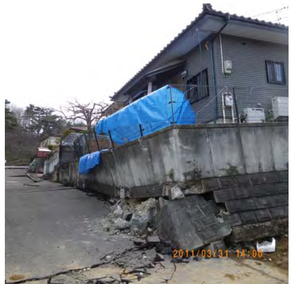
Fig. 9 Damaged residential fill in Sendai
