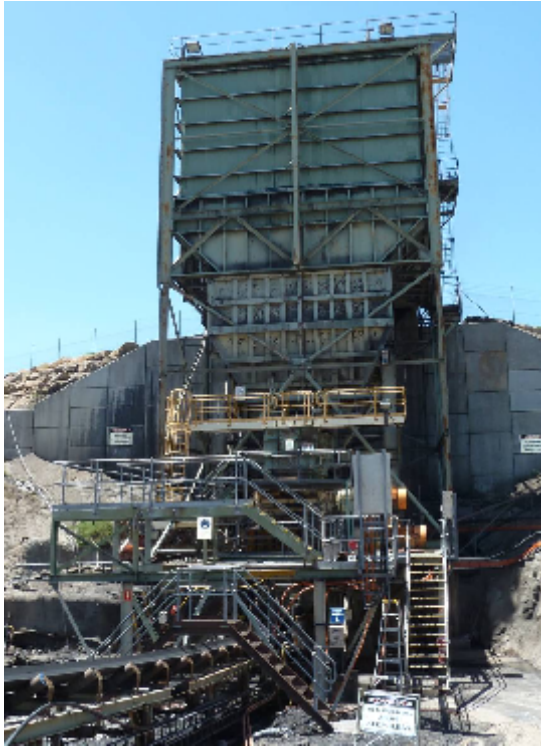
Figure 1: Geophones were placed on the ground at the base, at dump level (top of the retaining wall) and at the top of the structure.
