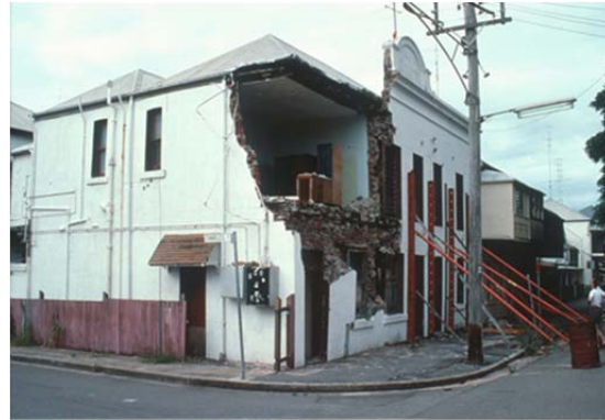
(b) Out-of-plane wall failure in the 1989 Newcastle earthquake
