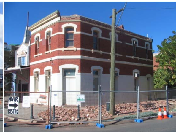
(d) Topped parapet in Boulder after the 2010 Kalgoorlie-Boulder earthquake
