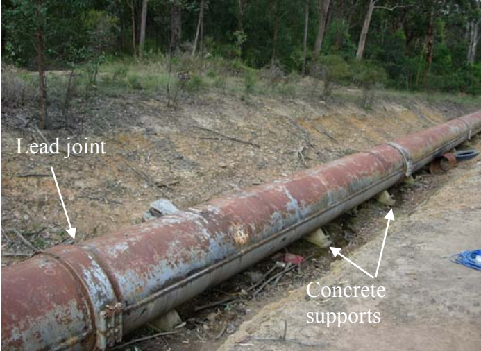
Figure 2: A photo of the pipeline showing the lead joints and concrete supports.
