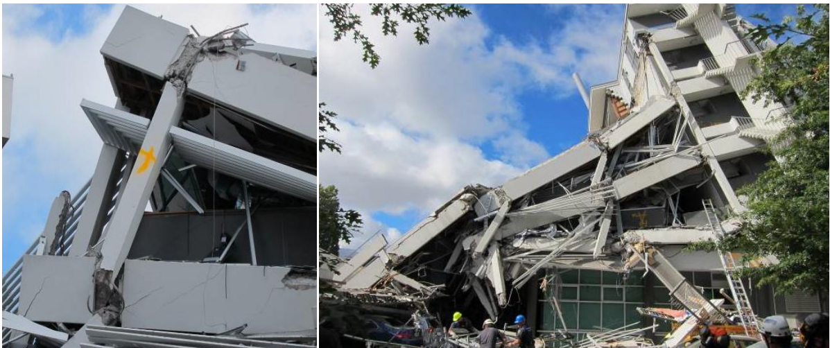
Figure 8. (a) Detail of joint failure in the Pyne Gould perimeter frame, (b) Collapsed Pyne Gould building from the northern side
