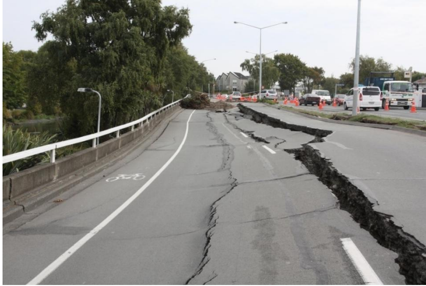
Figure 12. Effect of lateral spreading on the roadway
