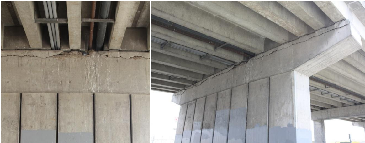
Figure 17. Crushing of the cover concrete in a bridge pier
