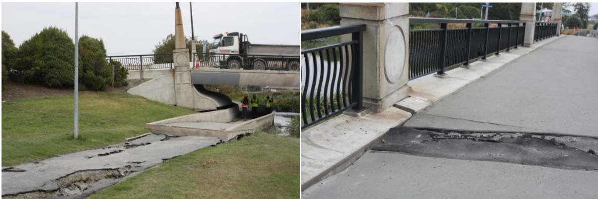
Figure 14. Rotation of bridge abutments and buckling of roadway
