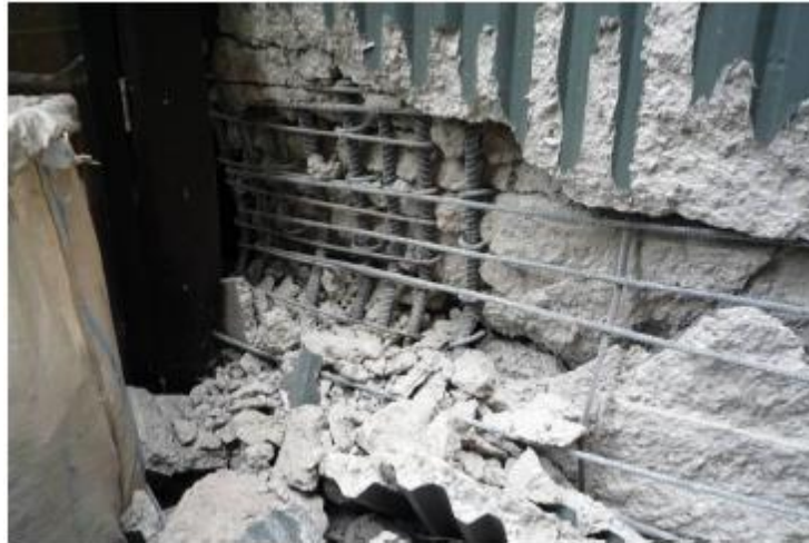
Figure 10. Compressive failures in walls. Loss of concrete and buckling of reinforcing bars in the plastic hinge zones
