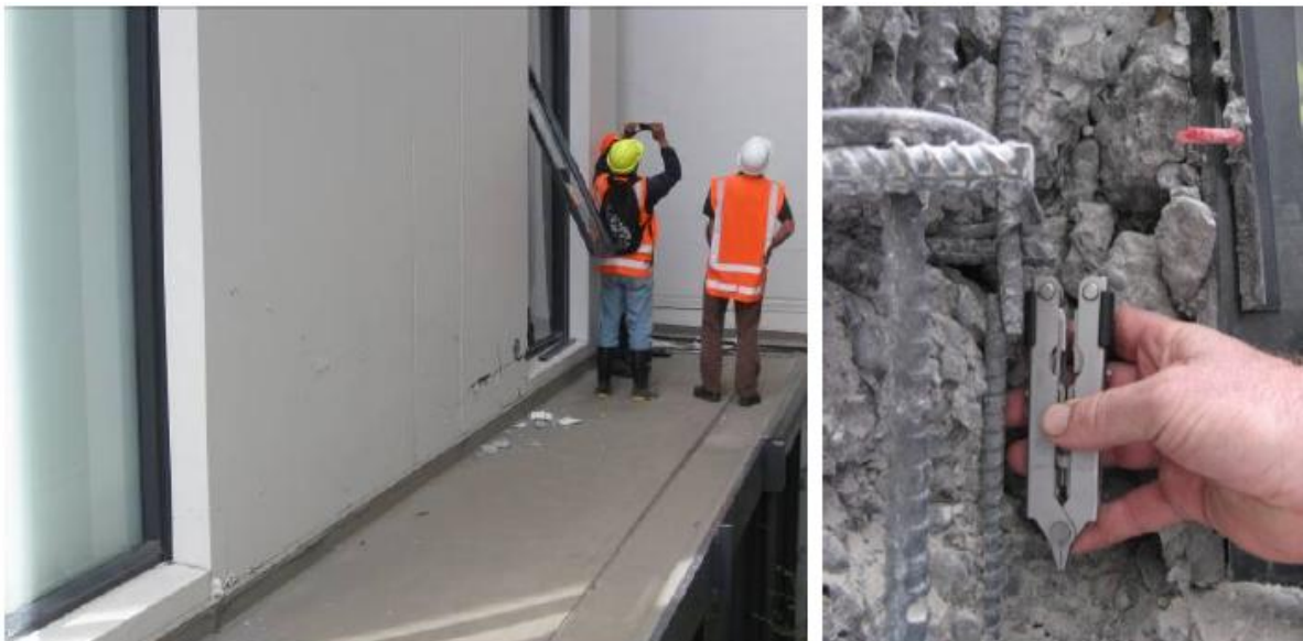
Figure 9. (a) Small cracks in base of a tall wall. Note the minor damage at far end of wall. (b) Damaged end of wall after breaking out some concrete. The vertical bars have yielded then fractured.
