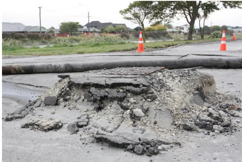
Figure 13. Flotation of pipe below causes the manhole to rise
