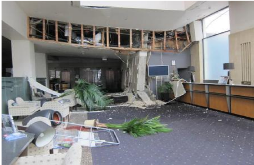
Figure 11. Collapsed Shear Wall in Hotel Grand Chancellor
