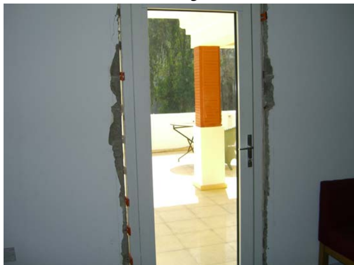
Figure 4: Rotary percussion drilled holes located too close to the masonry surface causing extensive spalling around perimeter of blast proof door.
