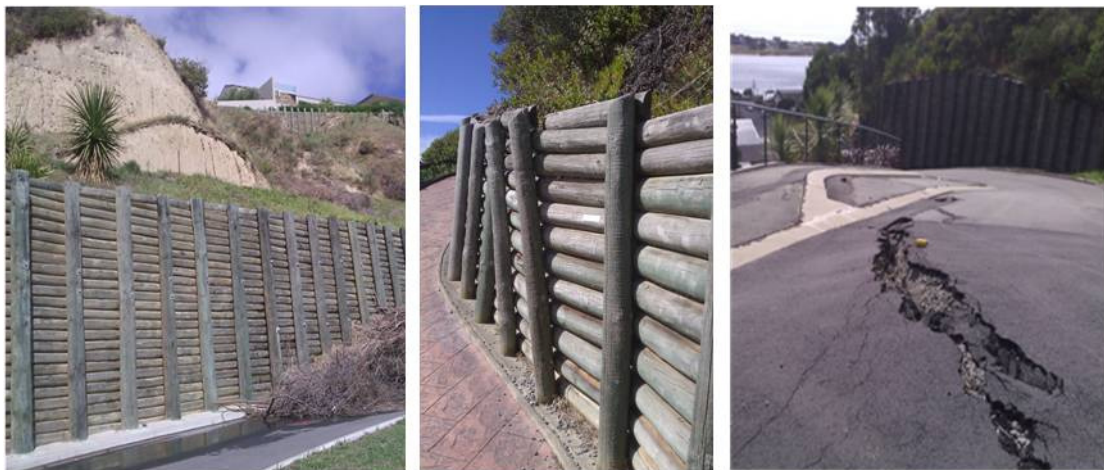
Figure 5: Timber pole walls (a) good performing timber pole wall with unsupported loess slope; (b) rotated timber poles; and (c) settlement of fill behind timber pole wall
