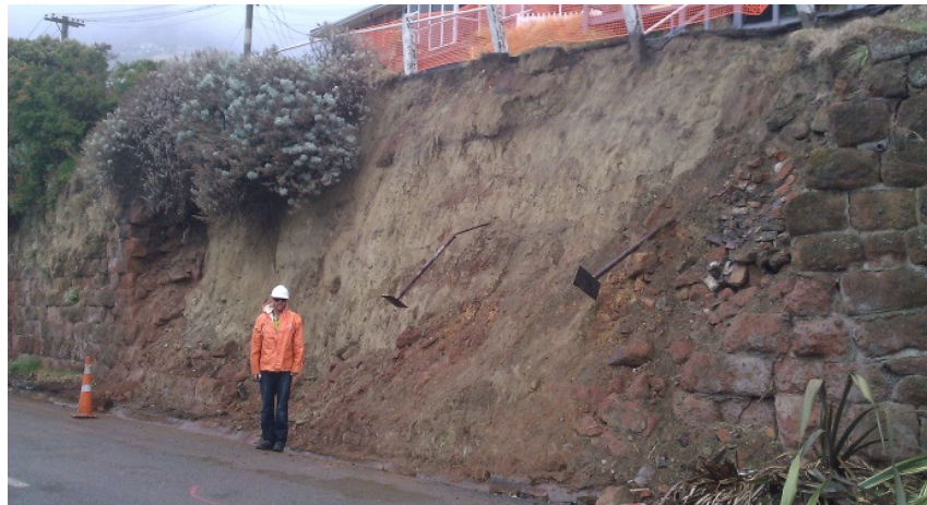
Figure 2: Collapsed Rock Wall and Free Standing Loess Slope in Lyttelton
