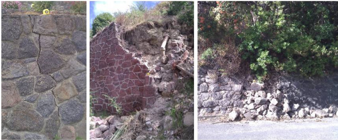
Figure 4: Rock Walls (a) cracks along grout; (b) structural collapse; and (c) toppled dry rock wall
