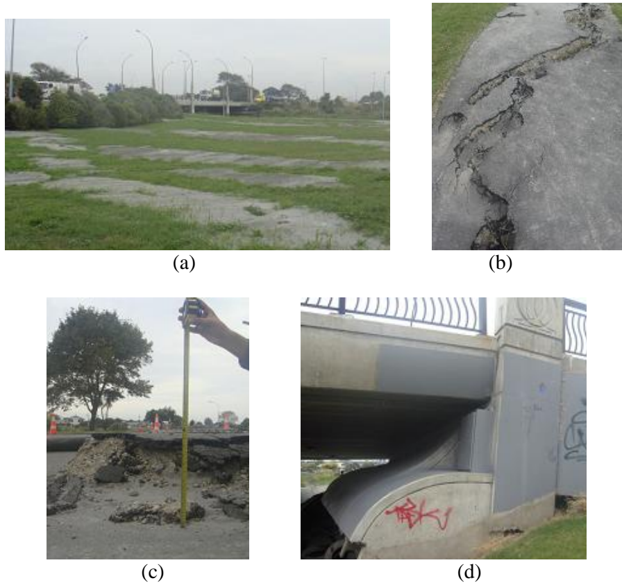
Figure 7: Damage to the ANZAC bridge and surroundings due to the 2011 Christchurch Earthquake: (a) sand boils on local site; (b) damage to walkway beneath the bridge; (c) relative ground movement around a manhole next to the bridge; and (d) damage to bridge abutment.
