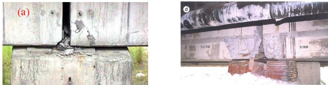
Figure 4. Typical pounding damage between bridge decks in Chi-Chi earthquake
