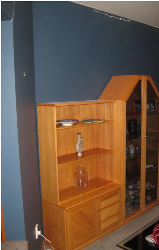
(a) Minor cracking
