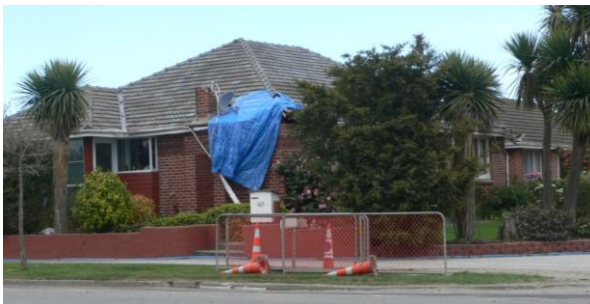
Figure 1 Collapsed unreinforced masonry chimney
